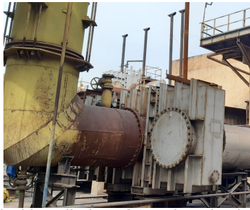
Fig. 2 Typical installation of Goggle Valve in gas piping main.
